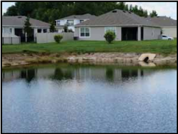
Figure 3 – Pond H Erosion
