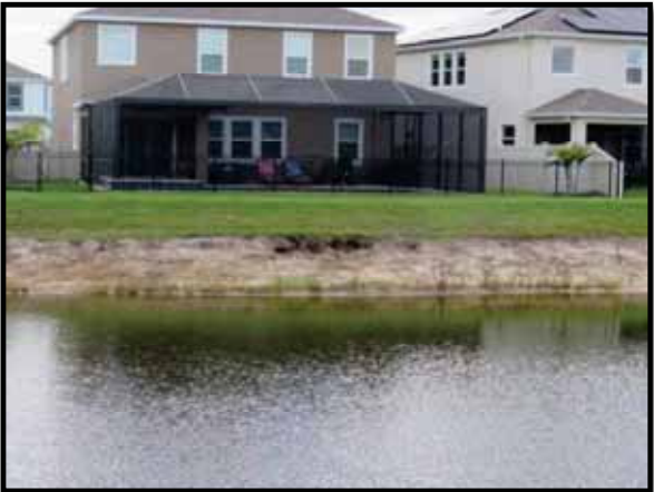
Figure 4 - Pond H Erosion
