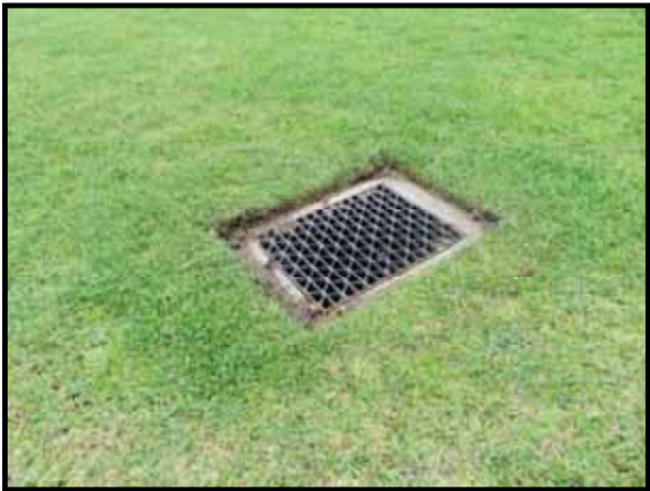
Figure 5 – Stormwater Catch Basin
